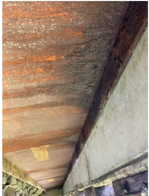
Superstructure - moderate rust scale
